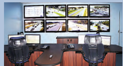
Traffic Management Center.
