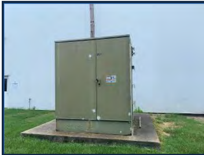
Photograph 13: Representative view of on-site pad-mounted electrical transformer.
