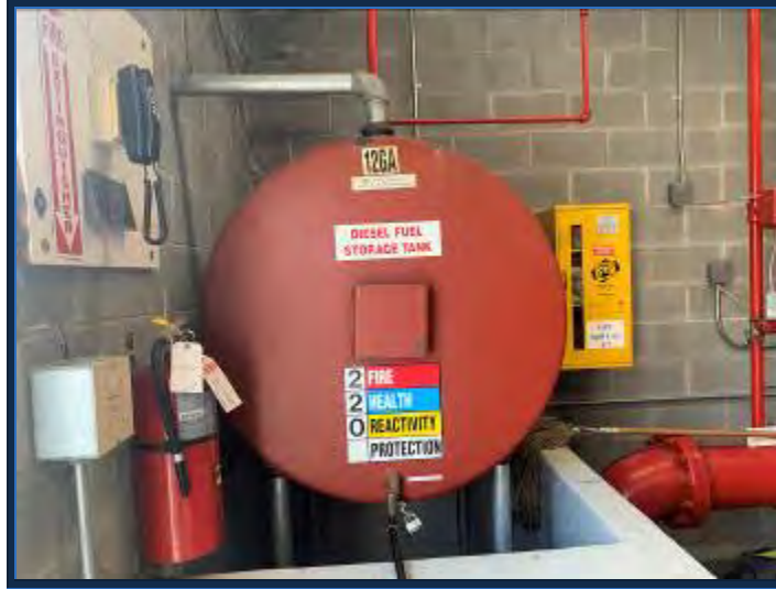
Photograph 10: Diesel AST in diesel fire pump house.
