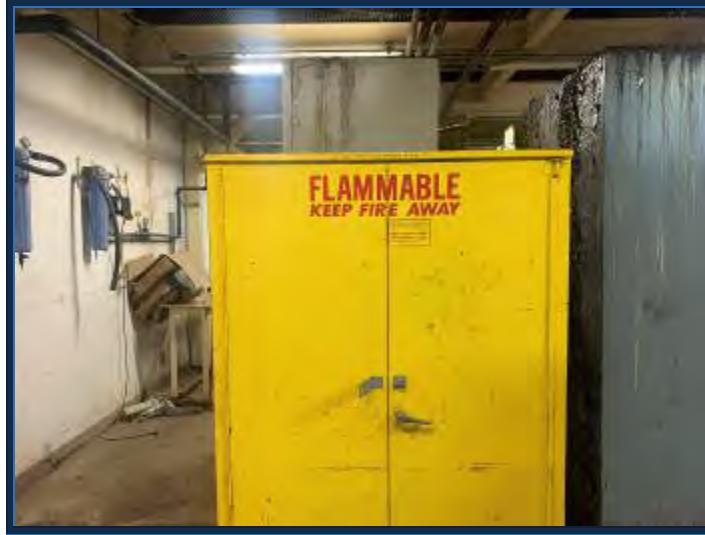
Photograph 12: Representative View of Flammable Cabinets.
